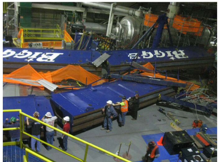
Power plant crane collapse. Image credit OSHA investigative report.
