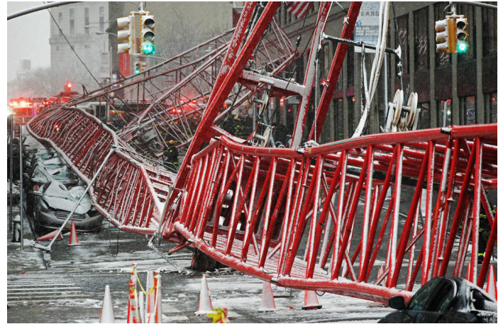
Tribeca crane collapse. Picture credit Milo Hess.
