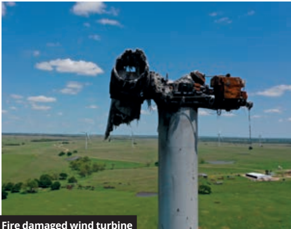
Fire damaged wind turbine
